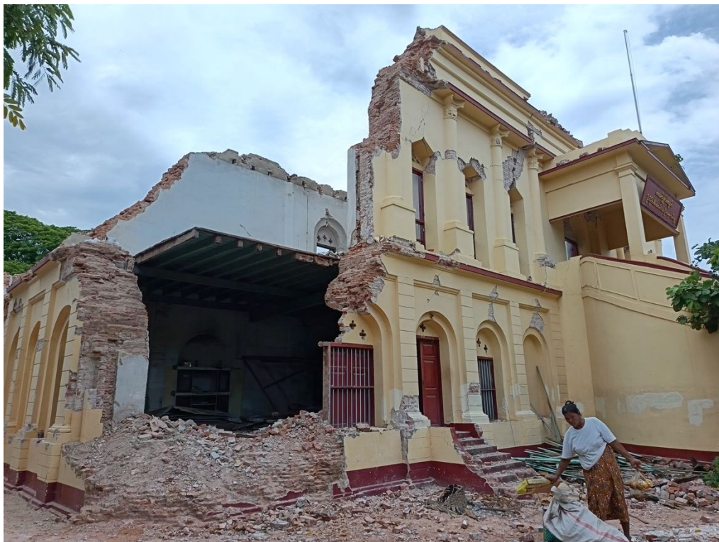
Figure 19 – Roof and walls of Maha Bandoola Monastery damaged by the earthquake, Mandalay (8 July 2025)
