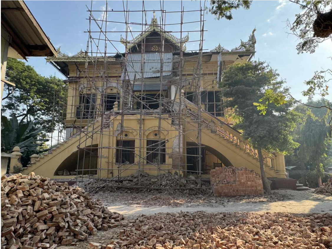
Figure 29 – Damage of the rear veranda of Abayarama monastery
