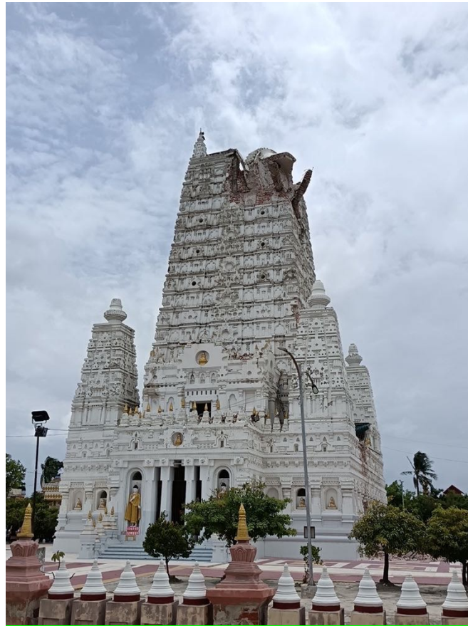
Figure 2 – Upper part of Mahabodhi damaged by the earthquake (8 July 2025)
