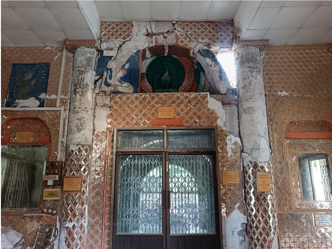
Figure 25 – Damage of glass mosaic, Shwe Yinye’ pagoda, Amarapura (15 July 2025)
