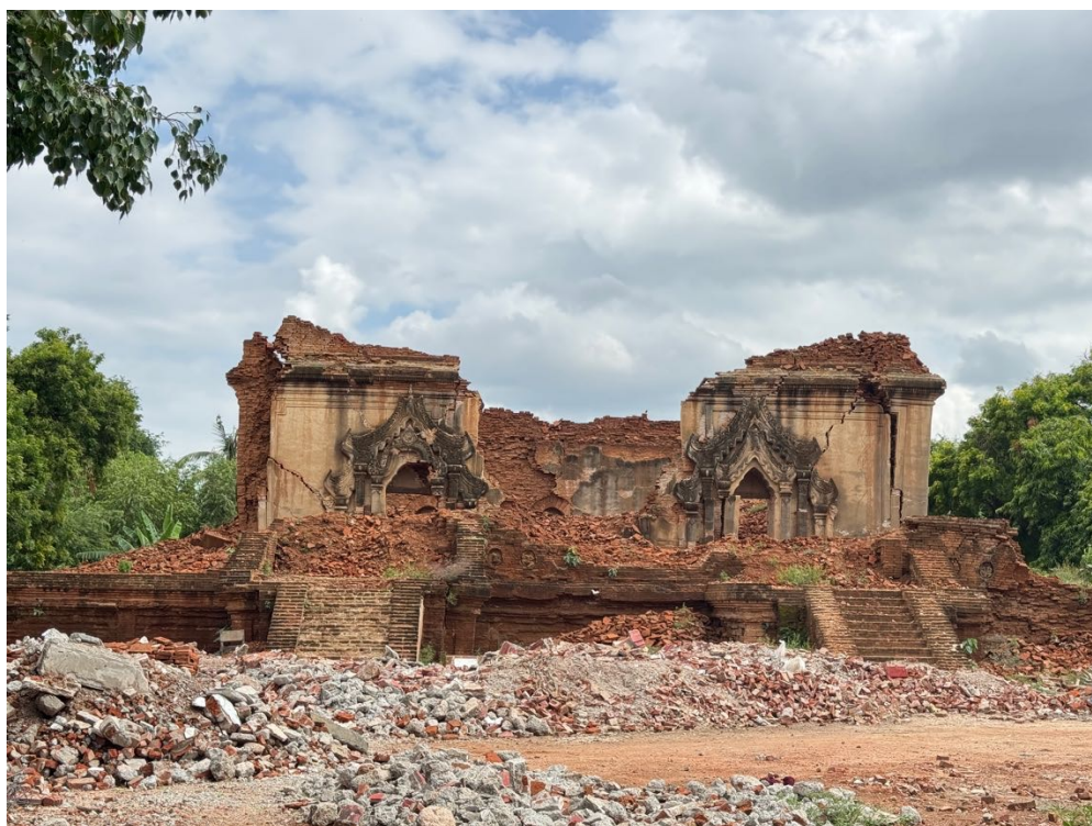
Figure 17 – Walls of Shweguyi Monastery damaged by the earthquake, Amarapura (17 July 2025)
