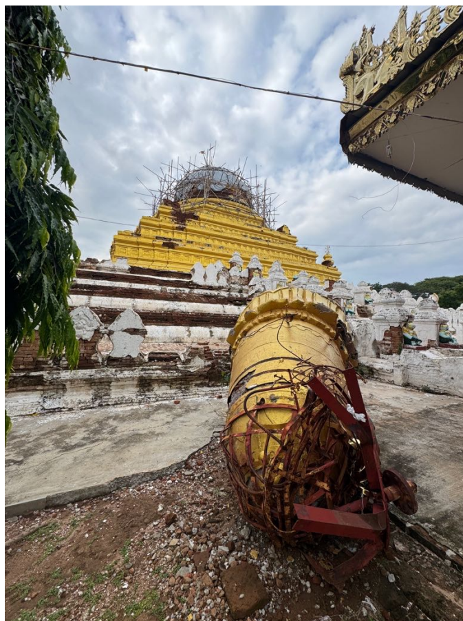
Figure 16 – Collapsed spire of Sandamuni Zedi, Amarapura (17 July 2025)
