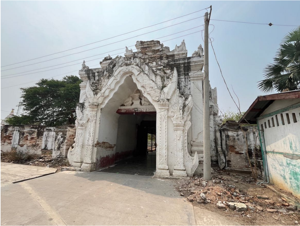
Figure 18 – Upper part of the entrance of Lawka Manisular pagoda damaged by the earthquake, Mandalay (1 April 2026)
